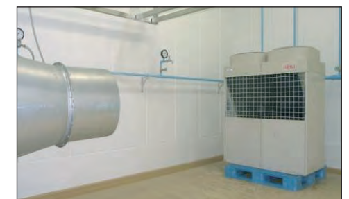
Shower Test Room
